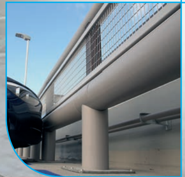
Minimal damage to floors
